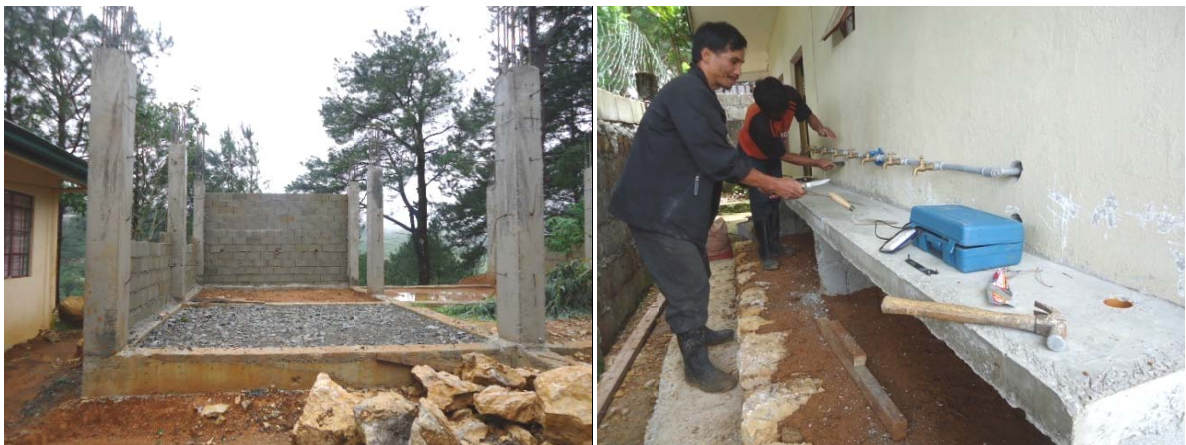
The ongoing construction of the Barangay multi-purpose hall (r) and the improvement of the Lubas Day Care Center adding a toothbrushing area for pupils (l).
