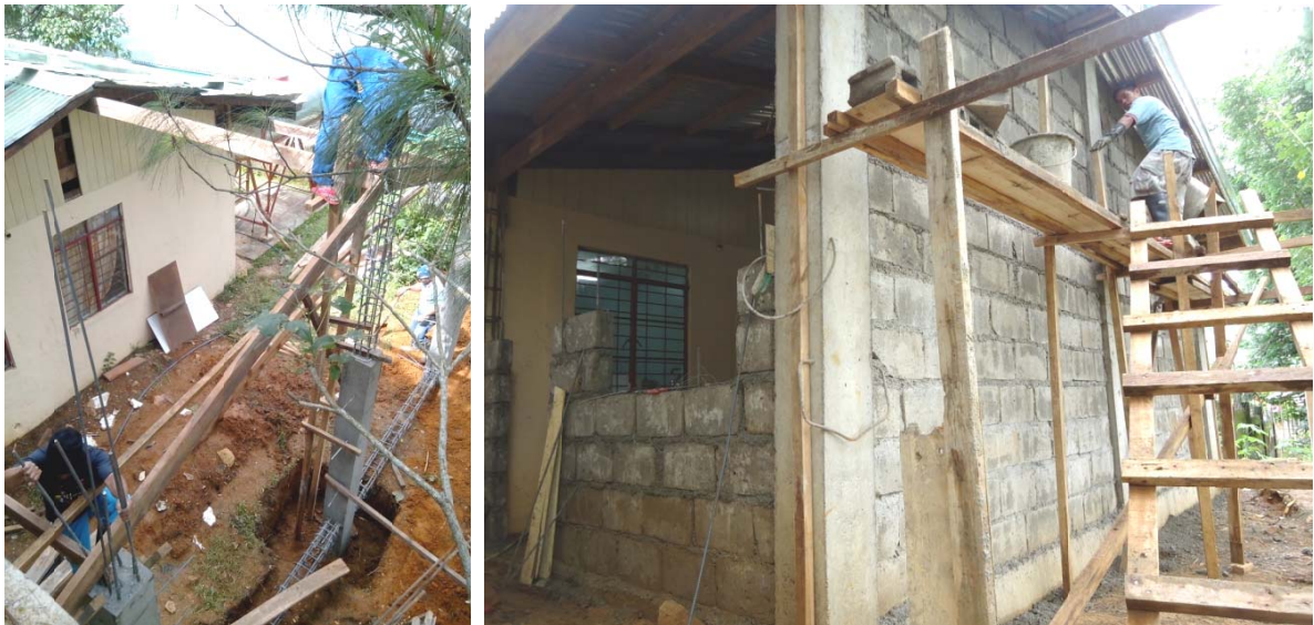
The ongoing construction of the additional two rooms at the barangay health center donated by the Korean-sponsored Children Development Program in Lubas.
